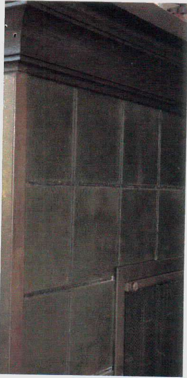
Detail of fireplace with ceramic tile, 1914, Oakland, CA.
